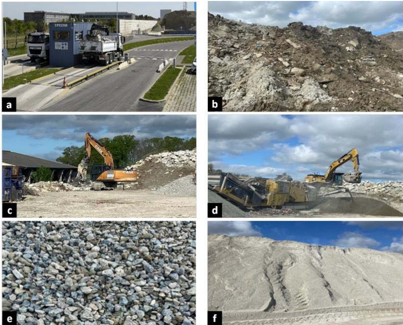
Figure16 Photograph of the YAM platform, a: Material reception and control station, b: Inert soil storage area, c: Crushing with a grab loader, d: Loading materials into the mobile crusher, e and f: Recycled materials
