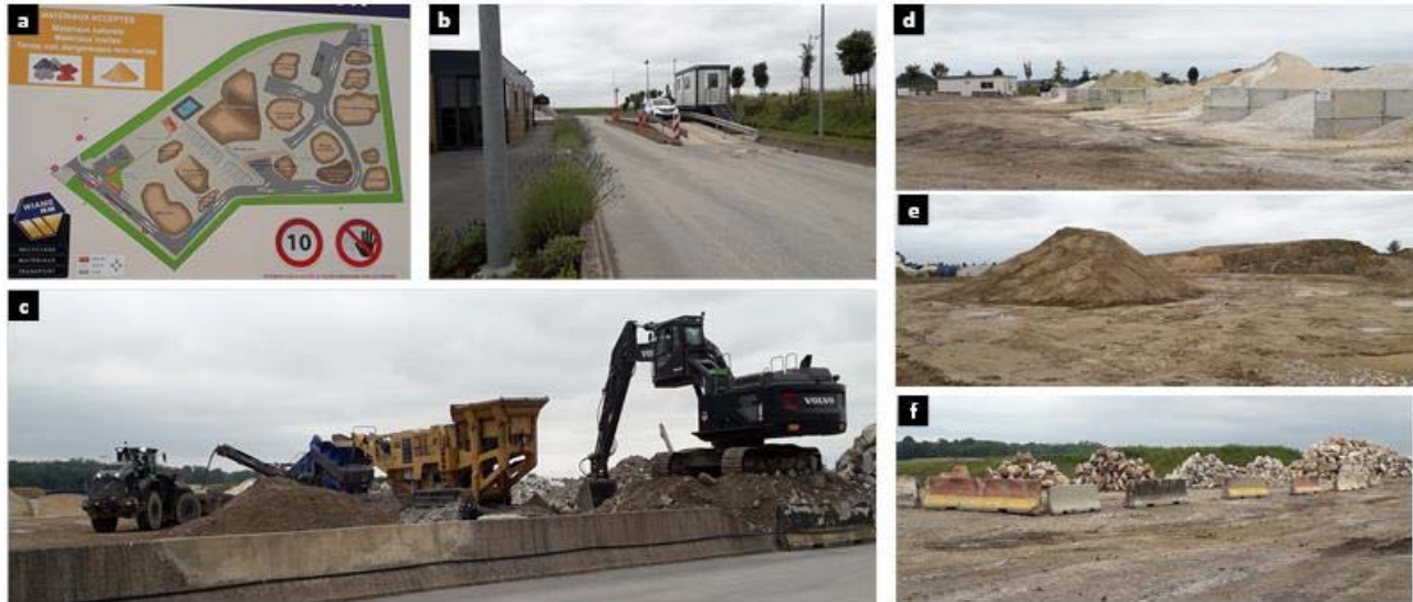
Figure 21 Photograph of the WIAME TP platform a) site plan, b) entrance with visual control and weighbridge, c) loader, crusher and screener, d) stockpile of recycled material, e) stockpile of soil (for limed soil), f) riprap and, at the rear, a mound of fertile soil (covered with vegetation).
