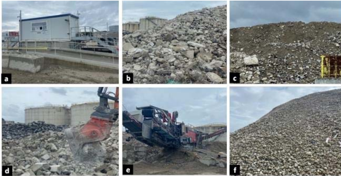
Figure 19 Photograph of the CEMEX platform in Gennevilliers; a: Waste reception and control station, b, c: Materials storage area, d: Materials preparation, e: Materials crushing, f: Recycled materials storage area.
